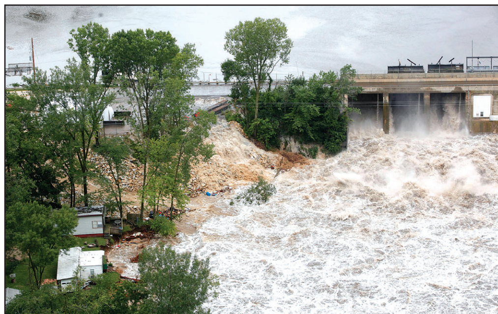
Maquoketa River water gushes out of the damaged Lake Delhi Dam on Saturday as areas surrounding the river in Delhi, Iowa, were evacuated.
